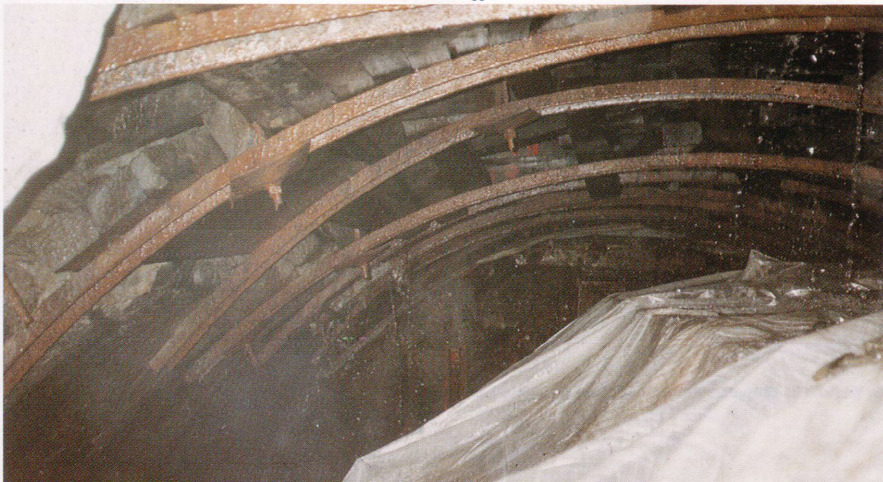
Ground support over the TBM was insufficient.
