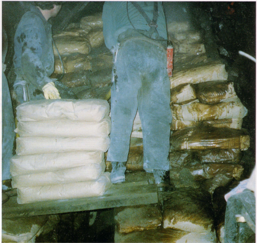
The relief drive was closed off using bagged cement which set in place.
