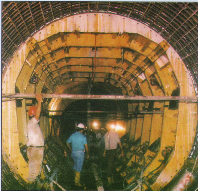
The picture shows the 4m diameter, 14m long, 290ft tunnel form built by EFCO for the deviation tunnel which is part of the El Diluvio Dam near the city of Maracaibo in Venezuela. The tunnel was constructed by Conintur, sub-contractor to the Seana-Omycca consortium. The 4m diameter, 14m long, 290ft form and its carrier were designed, built, and delivered from EFCO's Venezuelan factory.
